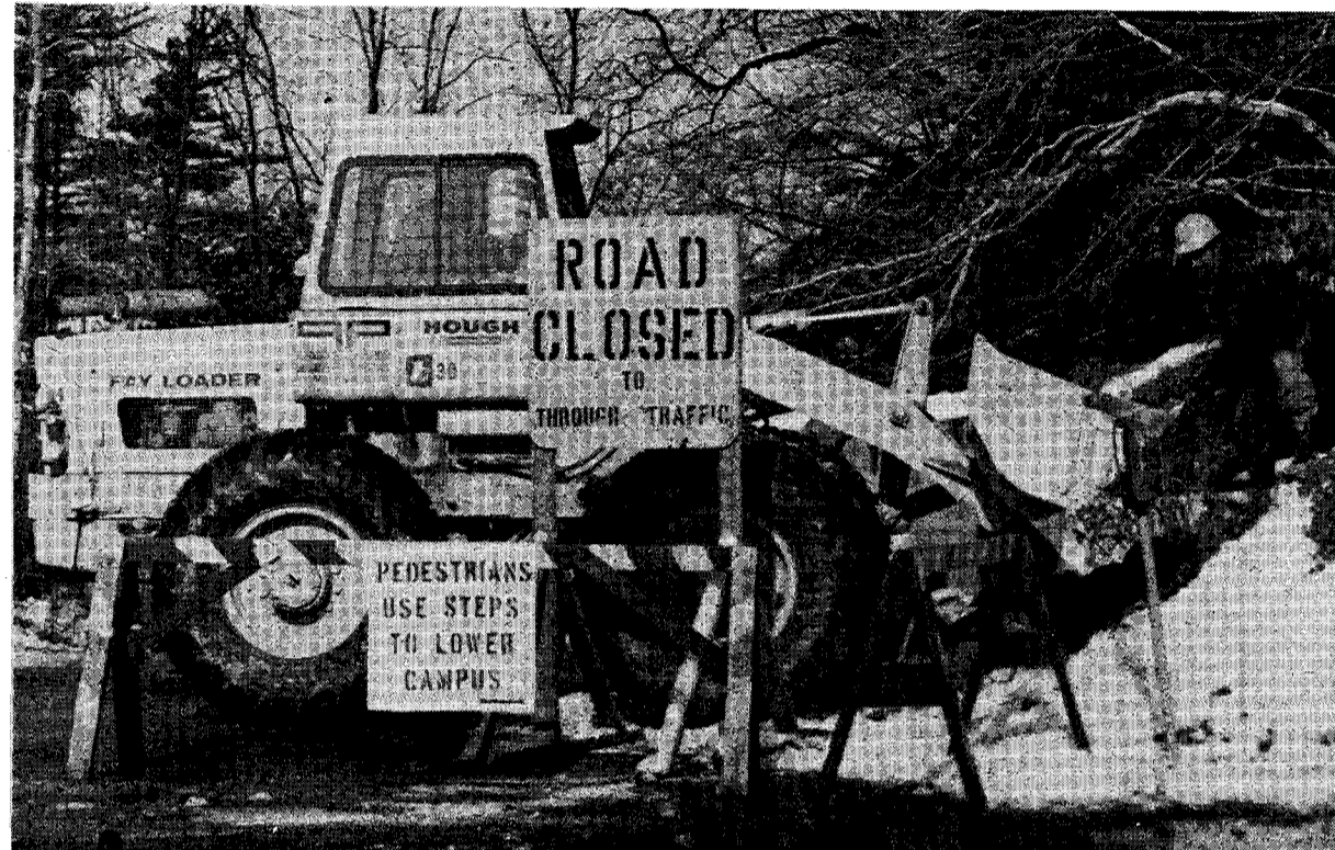
Well the big news on campus this week is that the _____ Pavement Co. is busily installing fox holes along the road into the valley of the Don and obstructing the passage of affluent day students who park their cars across the river. This construction was commissioned by the PRO TEM staff to provide defence against the of the Society of Liberals Urging Responsible Press. It is hoped that the road will be opened by Monday.
