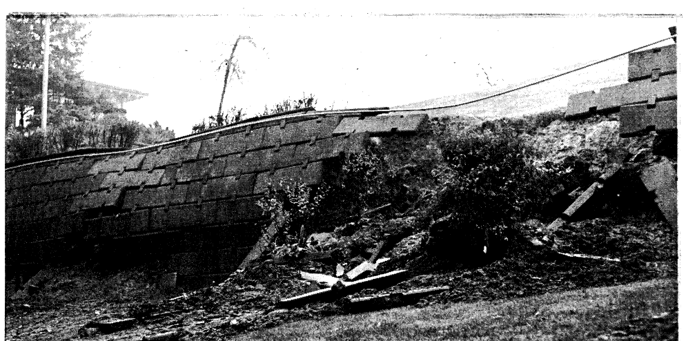
Campus Superintendent Andy Bevin described this section of the Rose Garden retaining wall as looking as if hit by a howitzer after it collapsed Monday morning.
